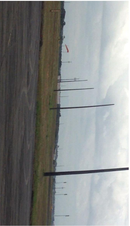
Existing Concrete Light Mast/Pole at the Remote Parking Area to be supplied and installed with LED Apron Floodlights and Obstruction Lights (Complete Fixture) together with their corresponding power feeder/supply, controls and mounting bracket.
